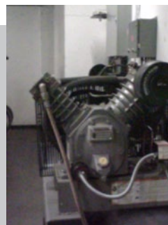
Air Compressor – Full Visible
